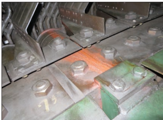
(a) Signs of excessive movement.
