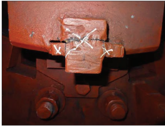
(f) Tangential crack on rotor radial key.
