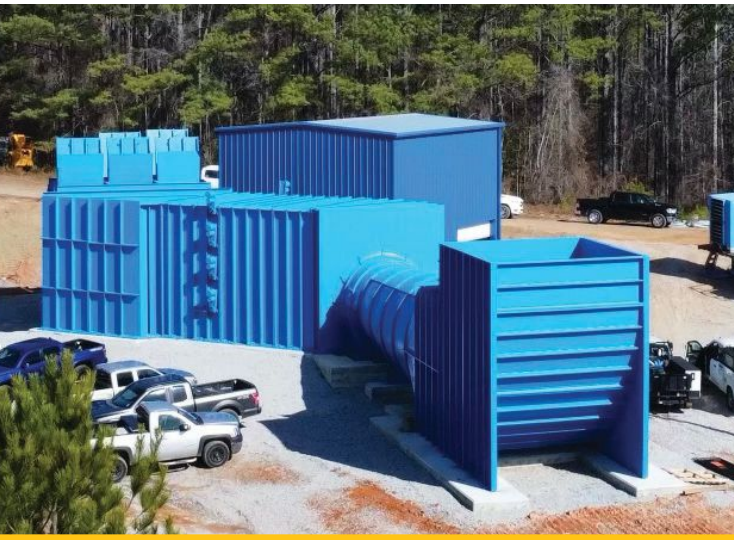
Mining operations present a moving target, challenging ventilation system design and operation. Photo: Paul's Fan
